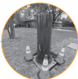
A picture of a cell phone tower under construction. Photo contributed by an ELi Reader
